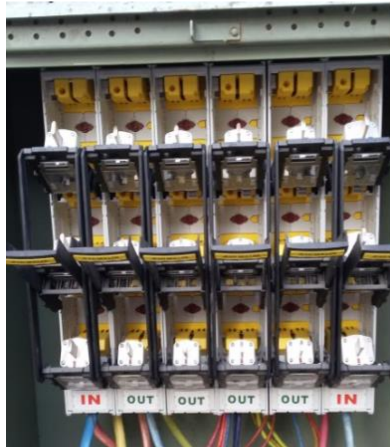
6Way Pillar Box, Switch open condition
